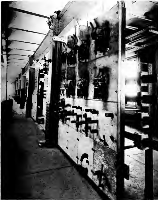
FIG. 9.—DIRECT-CURRENT AND EXCITER SWITCHBOARD.
